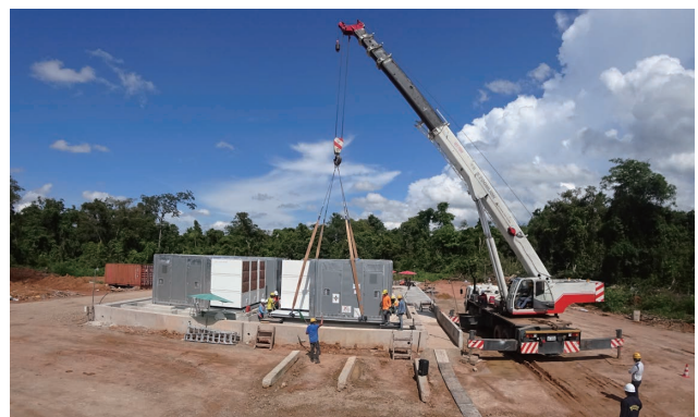
Figure 3: Installation of a Module by Crane Installation is completed in a few days, significantly reducing the construction period
