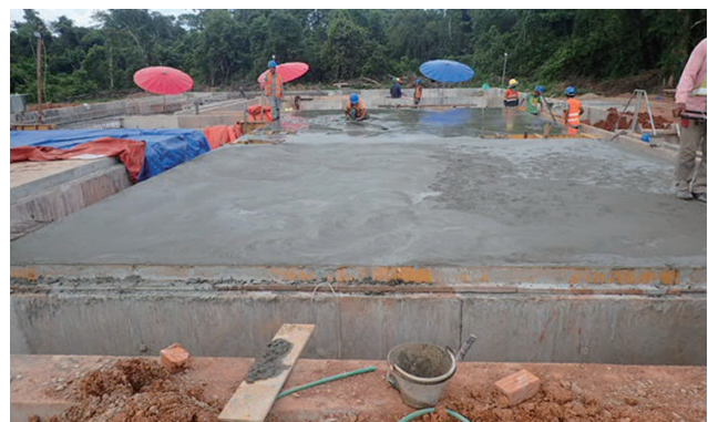
Figure 1: Construction of Concrete Foundations Creating shade with large sun umbrellas while working
